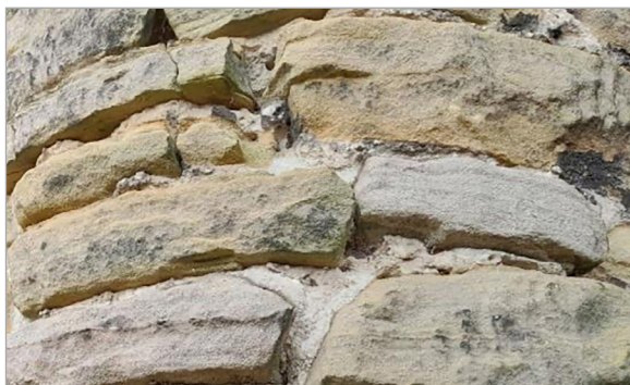
Missing mortar can lead to structural issues and water ingress if not maintained.
