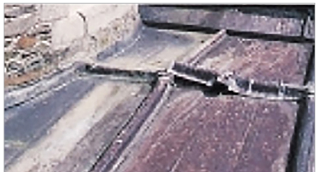
Splits in metal roofs or flashings should be repaired as soon as possible to prevent water ingress
