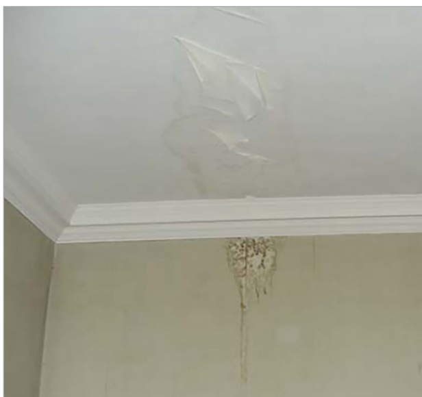
Water stains on internal walls indicate dampness in your property
