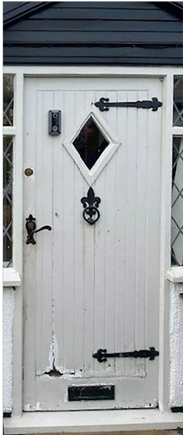
Repairing cracks or splits in door will also help reduce heat loss
