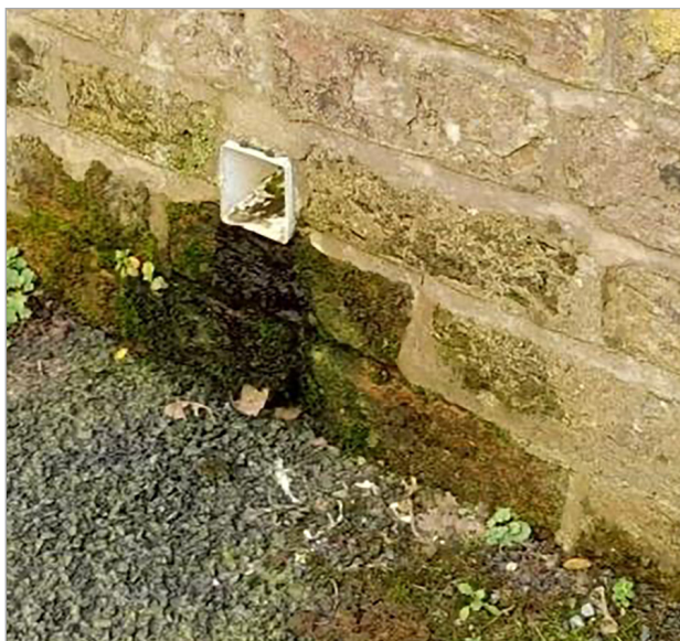
Moss and algae are an indication of dampness on external walls. Pipes should be extended to prevent this
