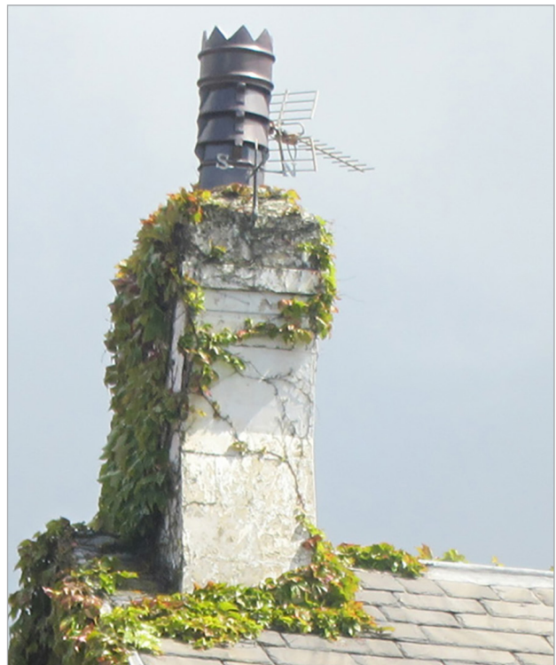
Plant growth should be removed to prevent moisture build-up
