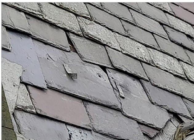
Missing or shifted tiles can allow water ingress causing damp inside the home
