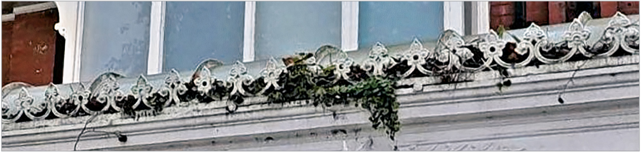
Blocked gutters cause water to overflow and can lead to issues with damp
