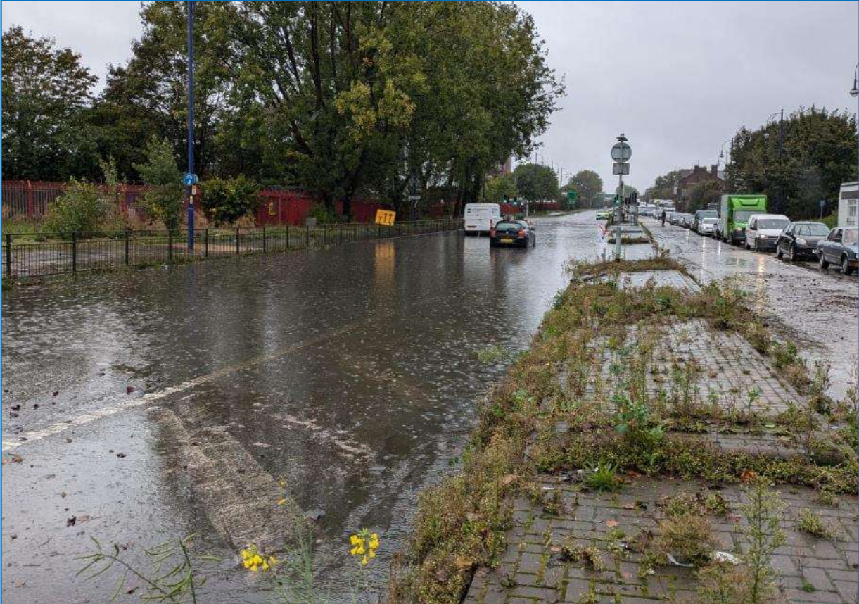
Figure 6: Flooding on Seaforth Road 30 th September 2024
