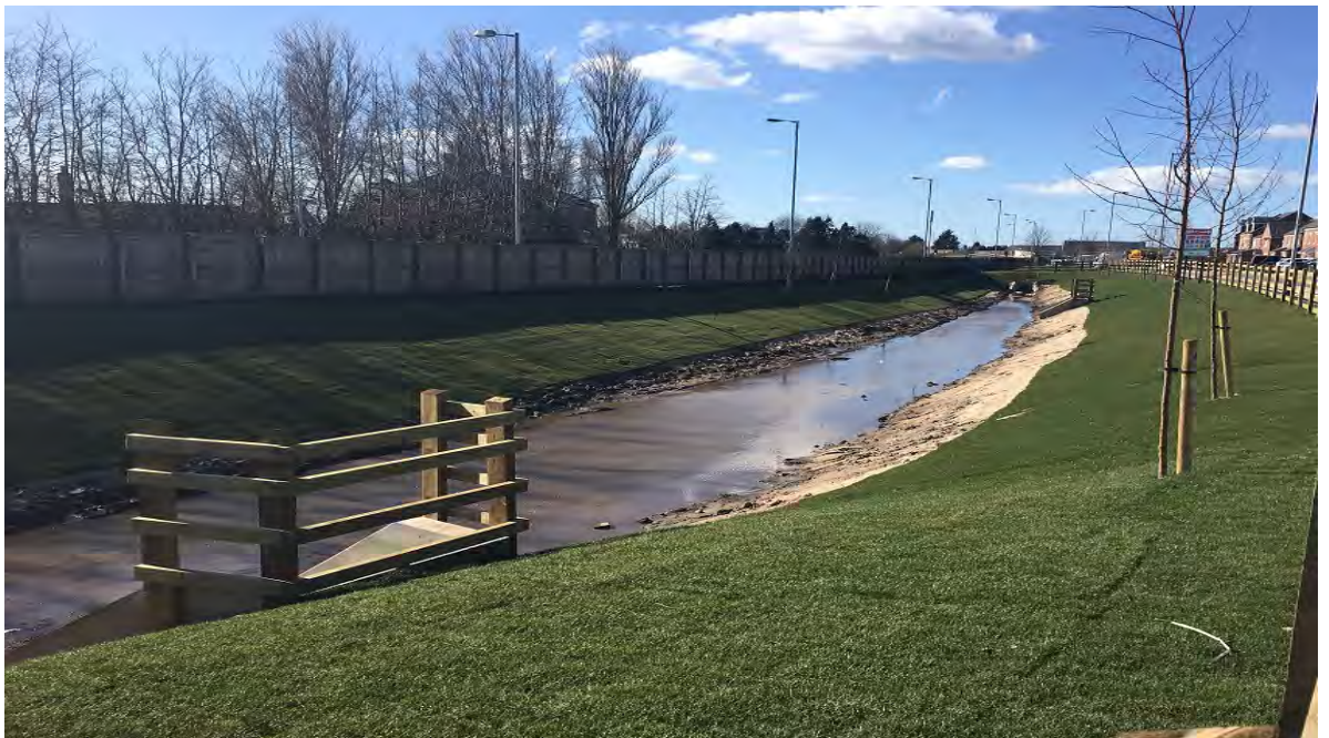
Swale (drainage system) – School Lane Poppyfields
